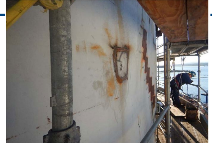
Pic. 1 – Shell distortion at insert.
