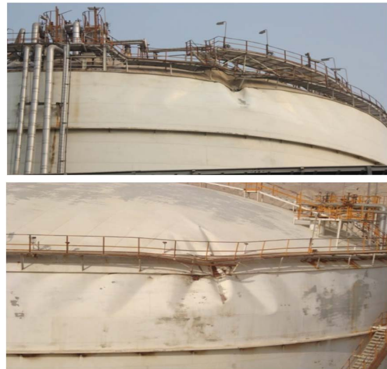
Reference: The Rupture of a Liquid Ammonia Storage Tank Study, Alireza Orooji and Sajjad Hosseininia, Assaluyeh, Iran
